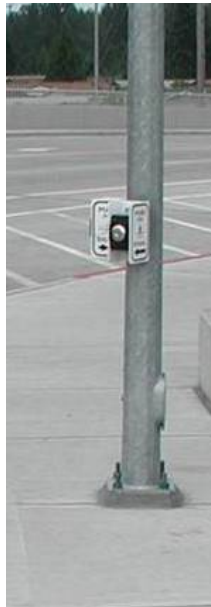
Typical Pedestrian Pushbutton
