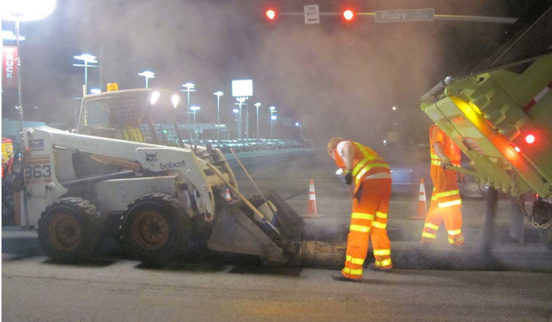
Maintenance patching pavement at an intersection requires significant planning, night work, and traffic control
