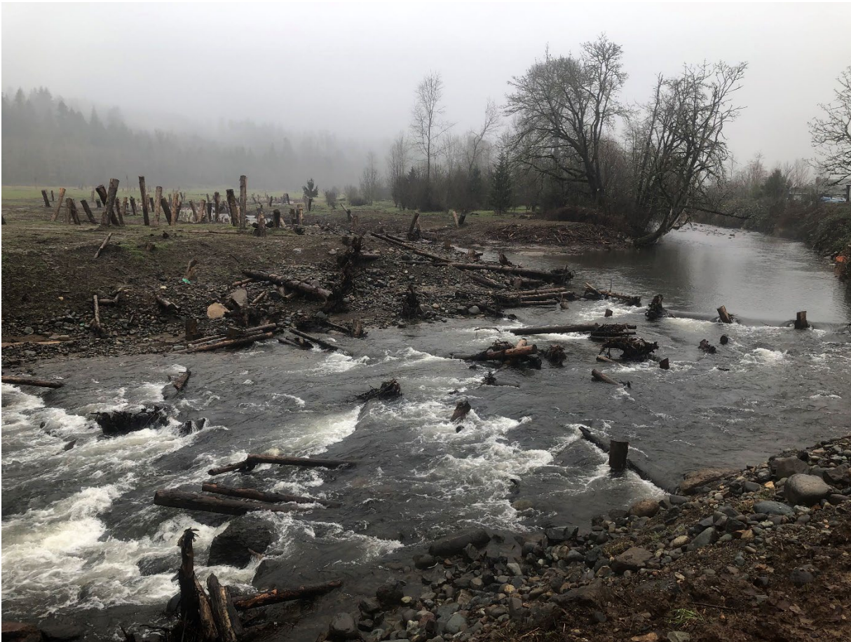
Figure 10-6 Example of Large-Channel Wood Grade Control
