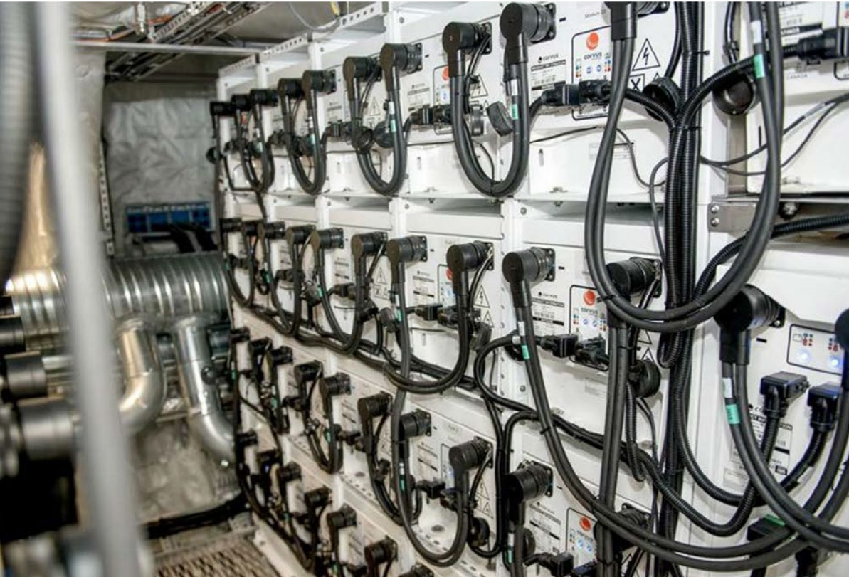
Cables connect to batteries in the battery room of the MF Ampere.
