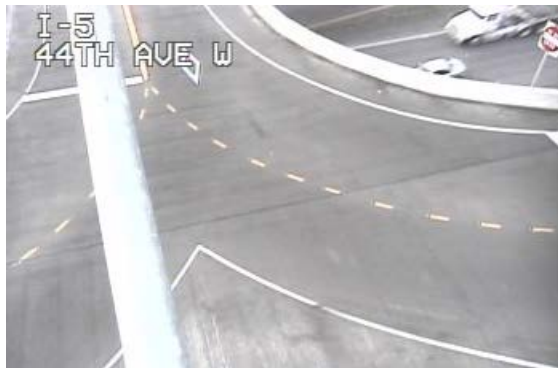
Guide striping provided for left-hand turns.
