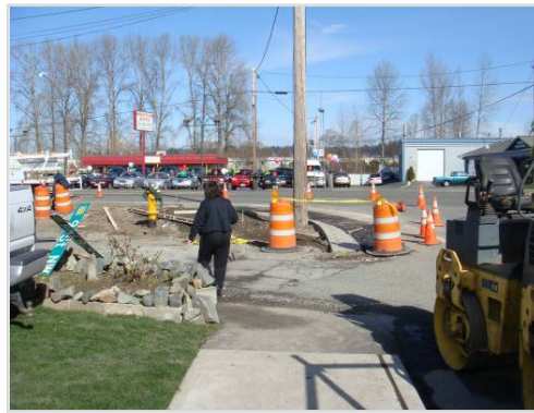
Does not meet ADA requirements
