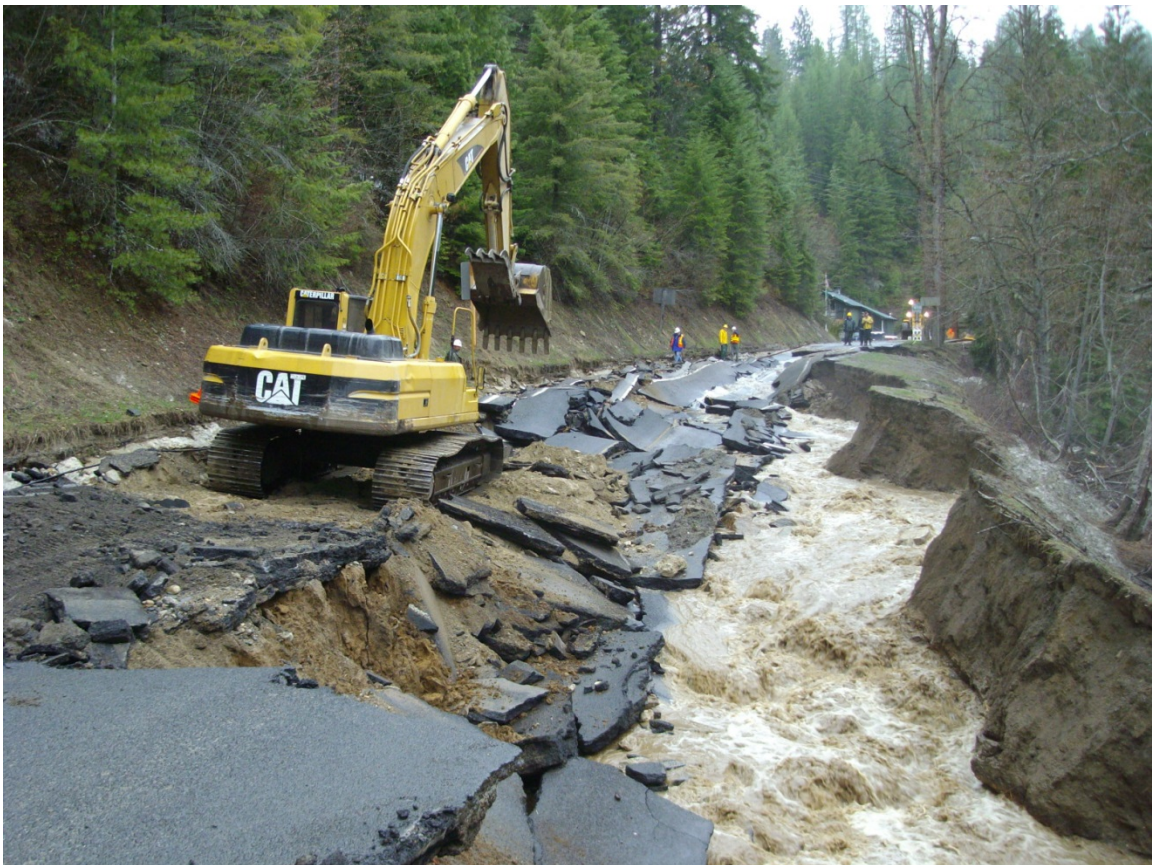
Maintenance responds to emergencies, which are more likely to occur during certain seasons
