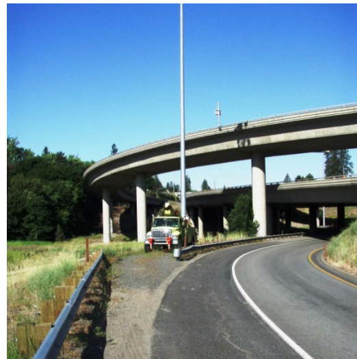
Well-designed access for luminaire maintenance
