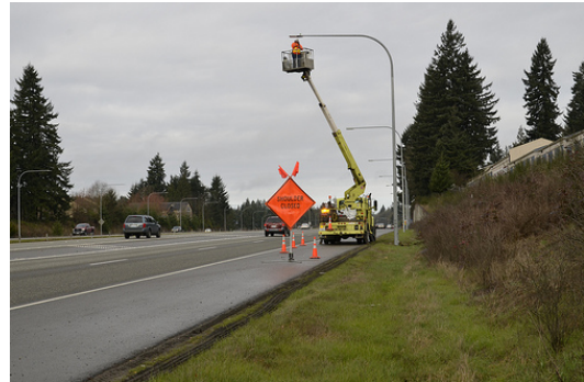
Access to maintain luminaire is provided through use of full shoulder
