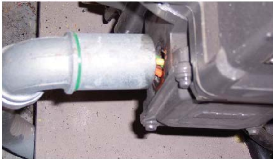
Photo 2 Broken conduit fitting on NE Thruster Brake
