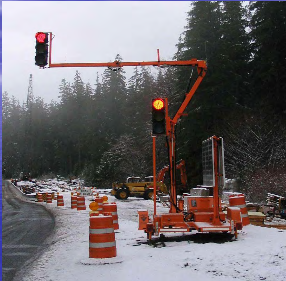
Portable Signal System
