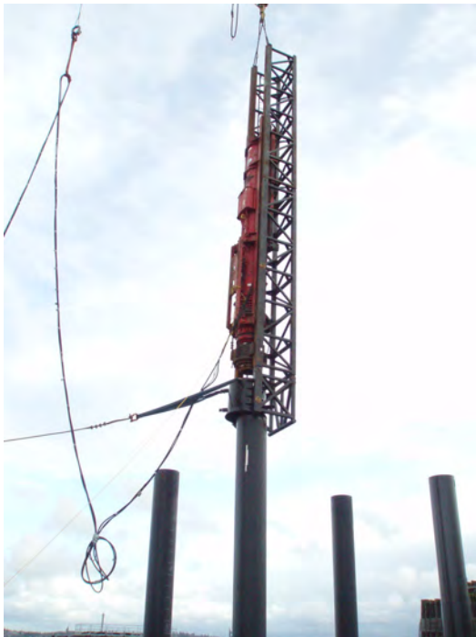
Figure 5. Photograph of 6,200 kg impact hammer being placed in position for pile driving at the Vashon Island ferry terminal.
