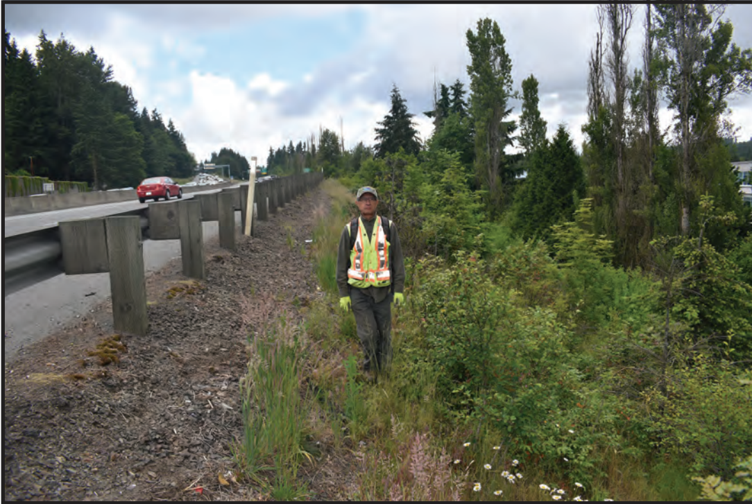
Exhibit 6-37. Overview of the fill slope immediately east of the I-405 northbound lanes in Zone 22, view is to the north. This area in Zone 22 contains a steep, 45-degree fill slope that could not be safely excavated. Crewmember is standing at the eastern boundary of the Limits of Construction.
