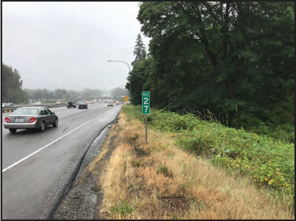
Exhibit 6-58. Overview of the fill slope immediately west of the I-405 southbound lanes at milepost 27, near the northern boundary of Zone 26, view is to the south. The fill slope is near Pit 20, which decreases in thickness with distance from 9th Ave and eventually transitions into intact native soil near the off-ramp.
