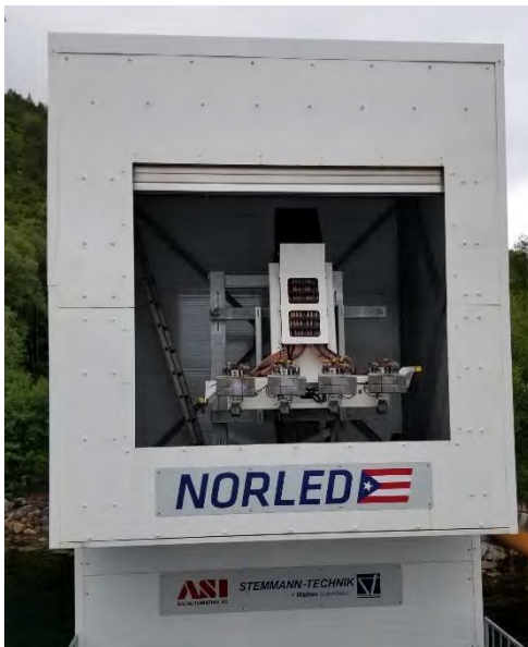
Figure 7: Stemmann-Technik First Generation Horizontal Pantograph RCS
