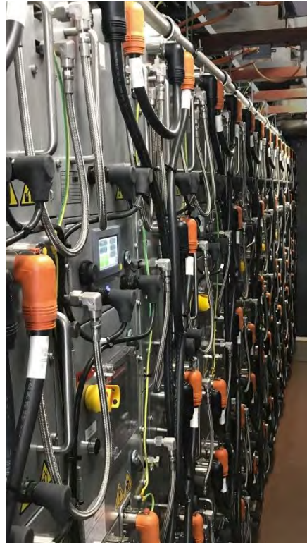
Figure 4: Sterling PBES (SPBES) Battery Racks
