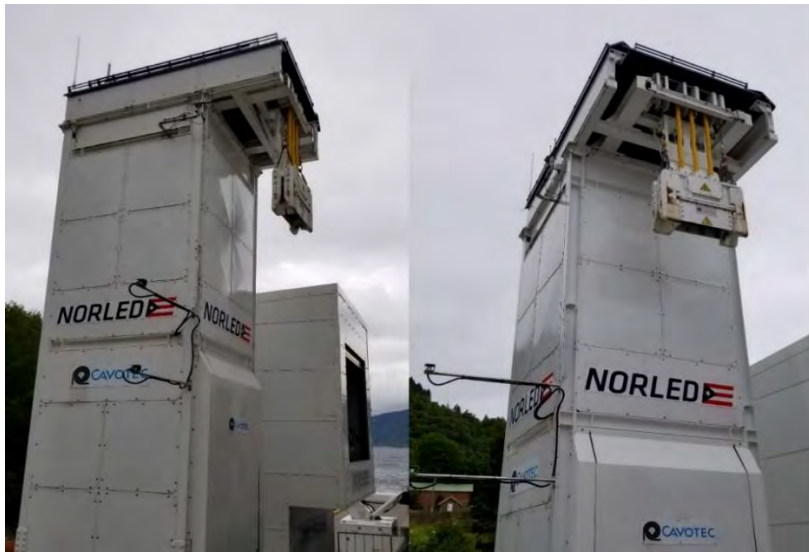
Figure 10: Cavotec APS Tower RCS
