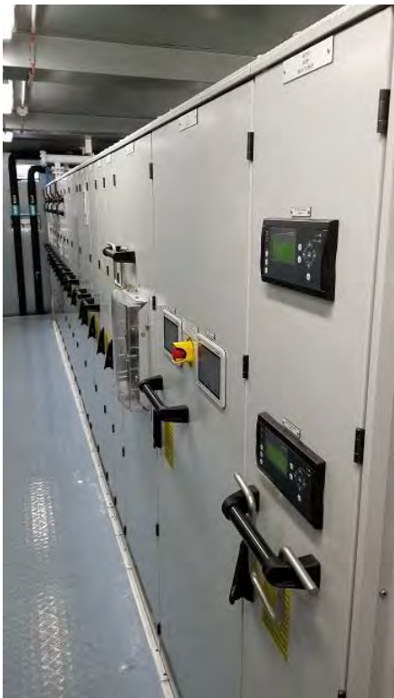
Figure 3: TYCHO BRAHE Shore Power Inverters
