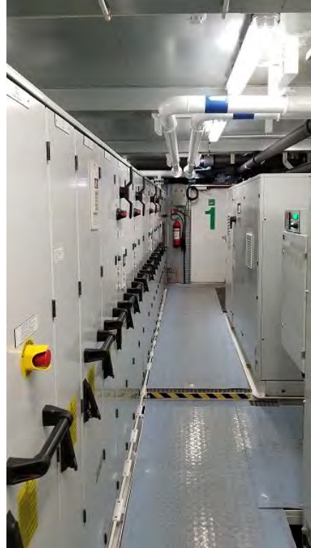
Figure 2: Interior of Converter Container
