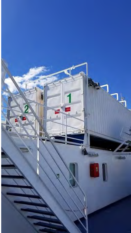
Figure 1: TYCHO BRAHE Battery Containers
