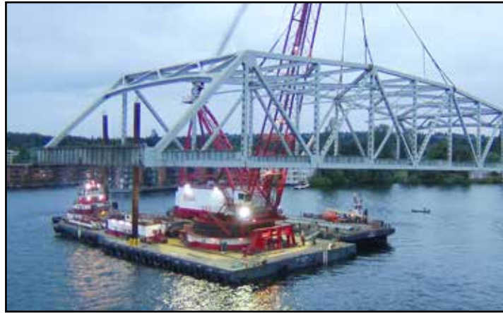
A derrick barge removes a metal truss from the old SR 520 floating bridge.
