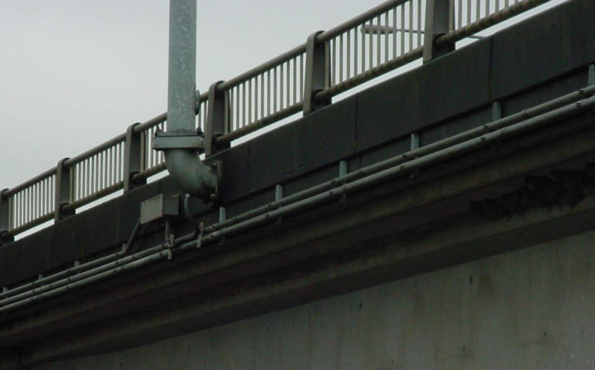
Conduit and Bridge Ell on Side of Bridge
